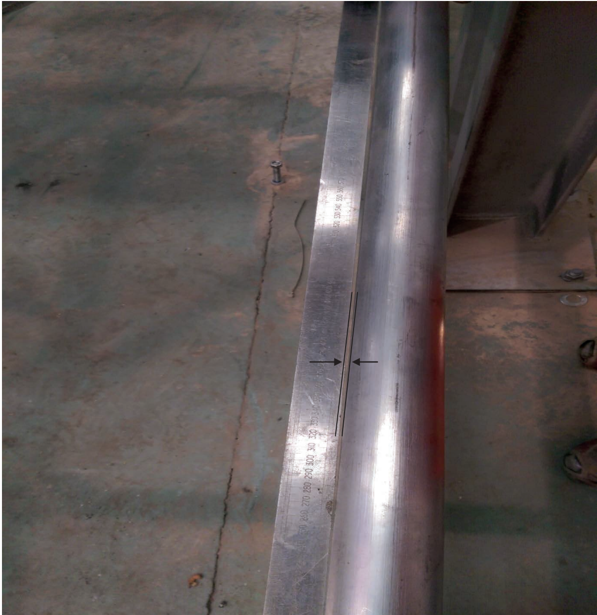
Permanent deformation of approx 3-4mm top chord post load
