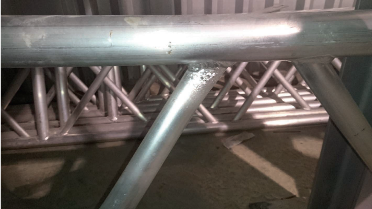
Figure 2.5.2. Side view of diagonal node compressive failure, note centre section buckling with no apparent visual weld defect evident.
