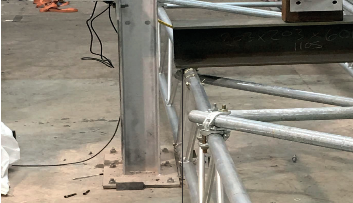
Beam vertical rotation noted.
