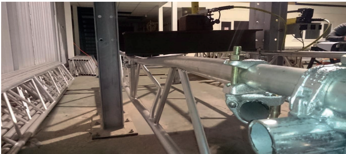
Figure 2.5.1. Digital image of diagonal node failure
